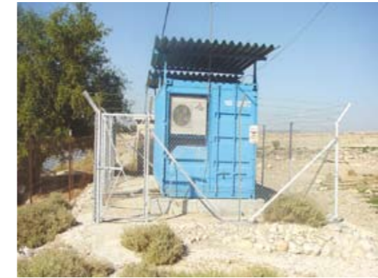
Monitoring station - outside view
